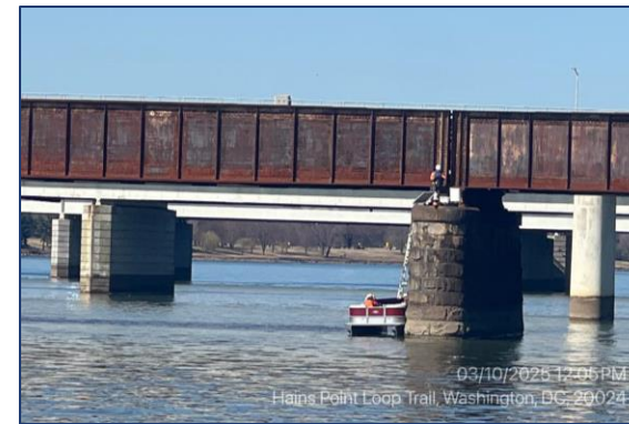
Devices to monitor vibration and settlement have been installed on existing CSX bridges over George Washington Memorial Parkway, the Potomac River, and I-395.
